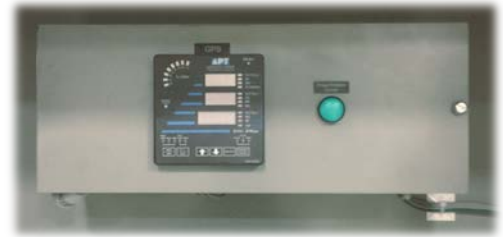
Figure 3: Power Quality Metering & Phase Rotation Indication
