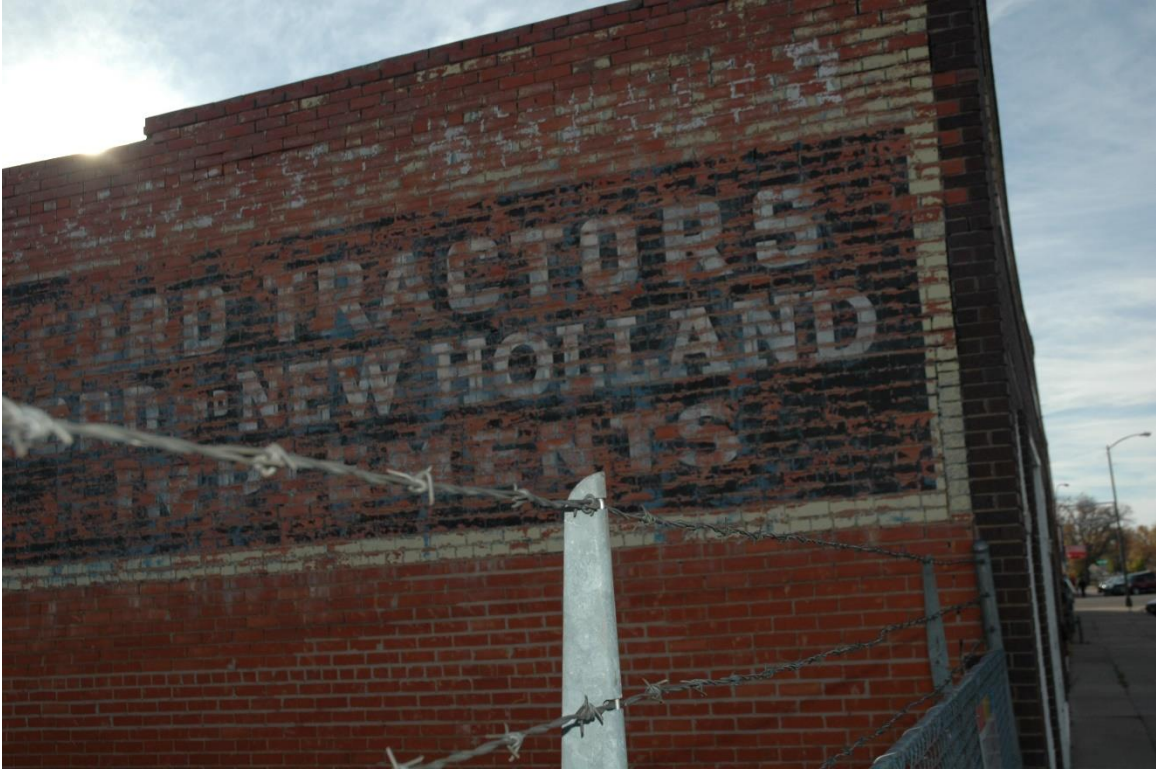
CD 1, Image 168, View to west of ghost sign at north end of the east-facing wall
