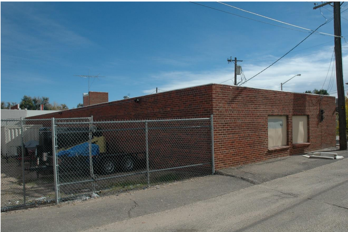
CD 1, Image 129, View to SE of rear (west) and rear portion of north side
