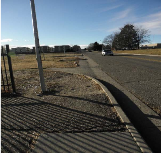
30th St. & about 20 th Ave – No sidewalk or ramps
