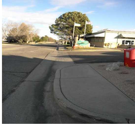
30 th St. & about 21 st Ave – No access ramps
